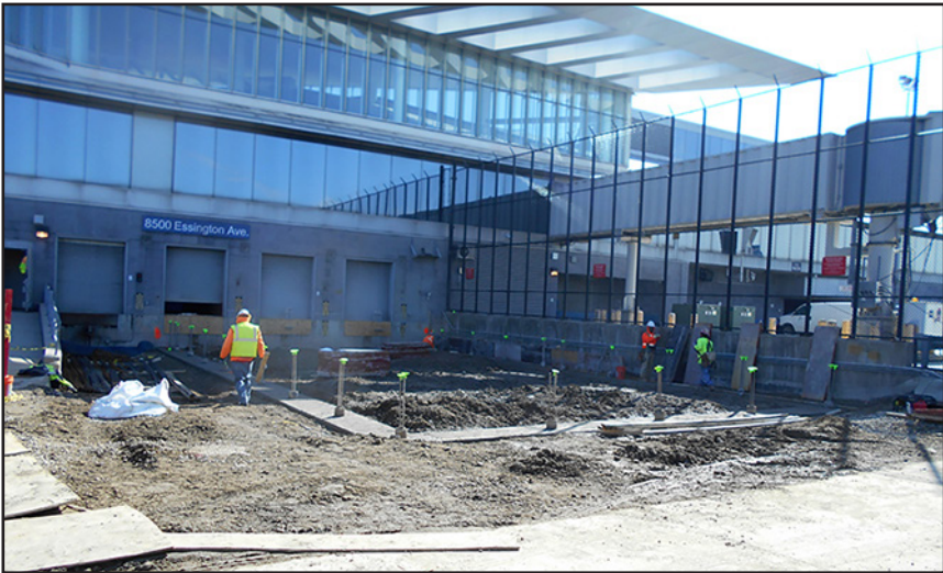
Construction Management Services on Terminal A West Sector 3 CBIS Baggage System at Philadelphia International Airport (PHL)
