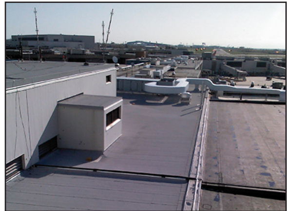
Construction Inspection B/C and C/D Connector Roof Replacement at Philadelphia International Airport (PHL)
