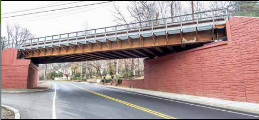
◀ Design-Build, Buckram Road Bridge Replacement Nassau County, NY Long Island Rail Road (LIRR)
