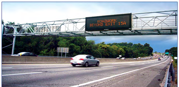
TANY-10-341 – Installation of ITS Devices at Various Locations in the New York Division [NYSTA]
