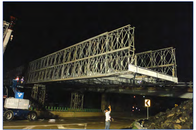
Rehabilitation of Rockaway Point Boulevard and Jacob Riis Pedestrian Overpass Bridges [TBTA]
