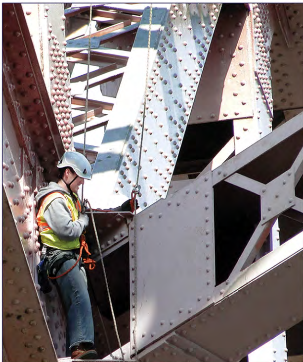
Hell Gate and Bronx Kill Bridges – Special Detailed Inspection and Rating [AMTRAK]
